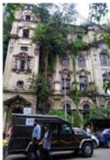
Massive plantations damaging the building
