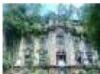
Oriental Assurance Building (1914), Uga- Office Plot No. 2, Olive Road, BBH Right (land value- very high) Ownership- LIC, Status- Protected Condition - dilapidated, trees have come up on roof
