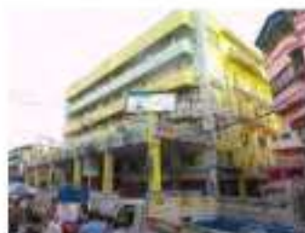
Guinea House (1917-21) Uga- abandoned Plot No. 131, Hornbair Street (land value- high) Ownership- LIC, Status- Unprotected Condition - Front facade mutilated, interior- retained
