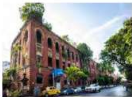
Large footprint, poor maintenance (left side), trees visible at top
