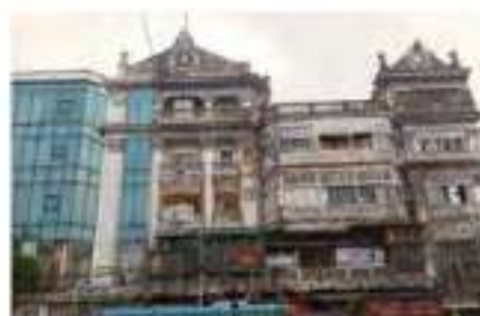
Opal Bazaar (1928), Uga- Residential/Commercial Plot No. 177B, C. R. Avenue (Land Value- High) Ownership- Private, Status- Unprotected Condition - Left side sold and the facade is mutilated with structural clearing
